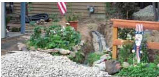
The area within 5 feet of your house is important to both water quality and defensible space concerns. When constructing erosion-control BMPs in this area, such as the installation of an infiltration trench shown at left, contact your local fire professional and Conservation District for advice on defensible space and BMPs.
