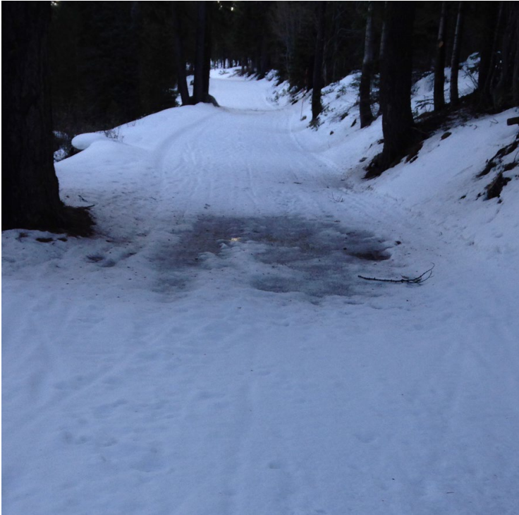
Safety Hazard on road into Euer Valley
