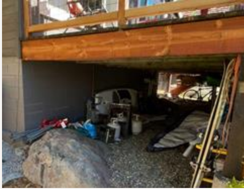
Before and After: Combustible stored under stored under deck cleaned up to remove ignition materials & propane tanks.
