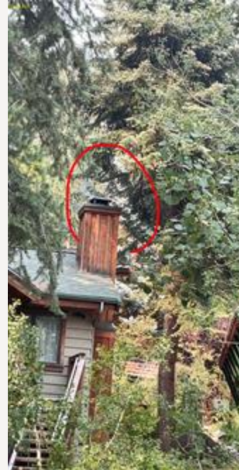
Before and After: Vegetation close to structure and overhanging roof.
