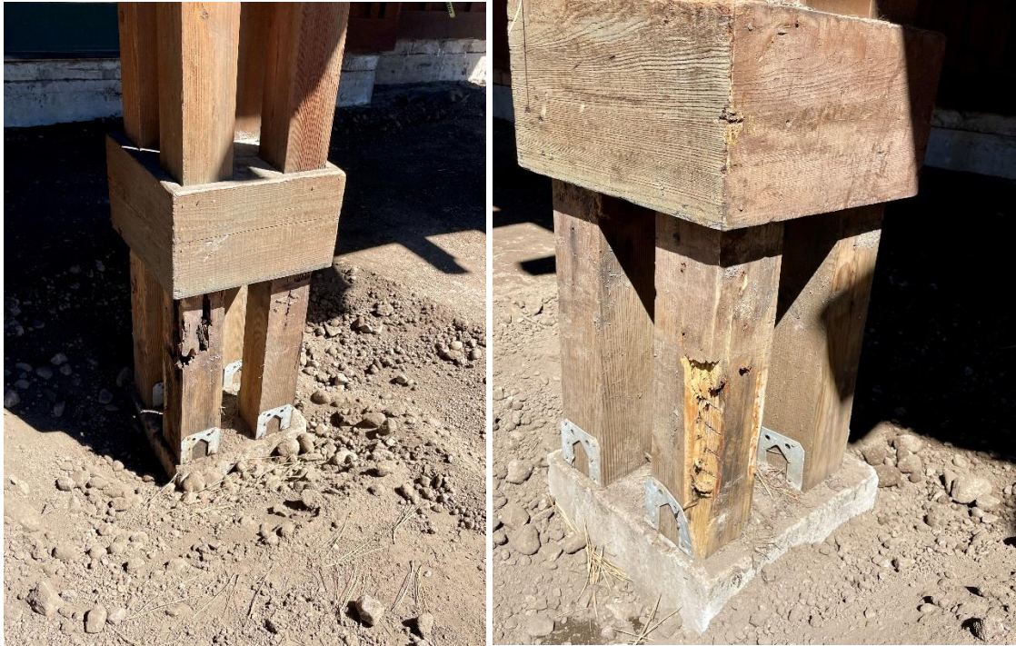
Column bases with rot
