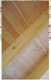
STRUCTURE + SOFFIT: DF GLB. 3x6 T+G VG SQ EDGE, NO GAP, CLR STAIN
